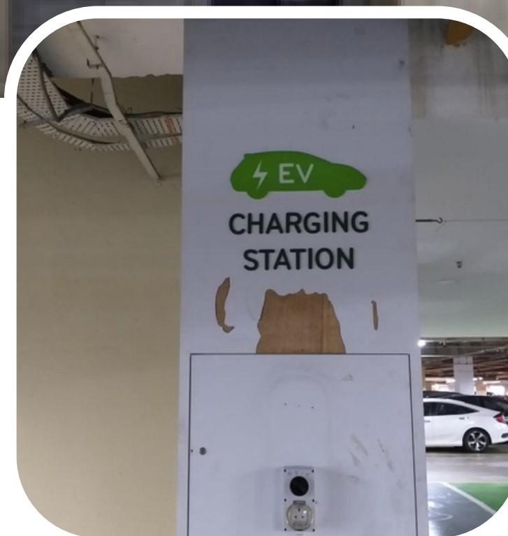
Car charging station is next to the lift
